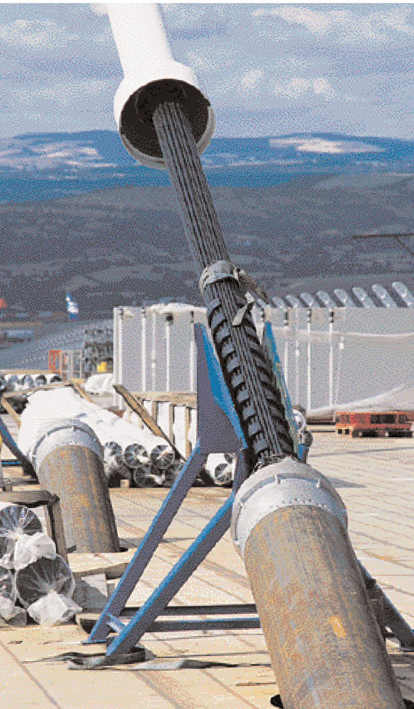
DURING LAUNCHING OF THE DECK , 24 stay cables installed on pylons P2 and P3 were used as launching cables. Temporary saddles placed on the deck and pylons helped to limit angular deformations in the anchoring points.
